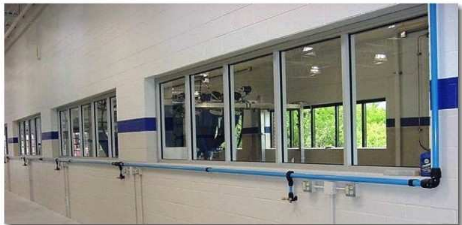
Air Piping System
