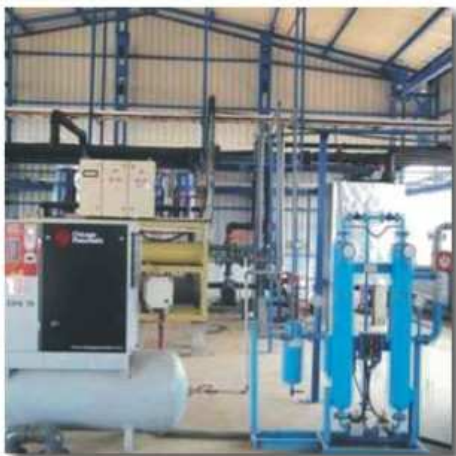
Compressed Air Piping System
